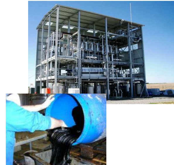
Acid organosolv Pilot plant ARD
